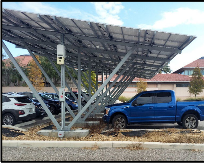
33. USF solar panel parking area
